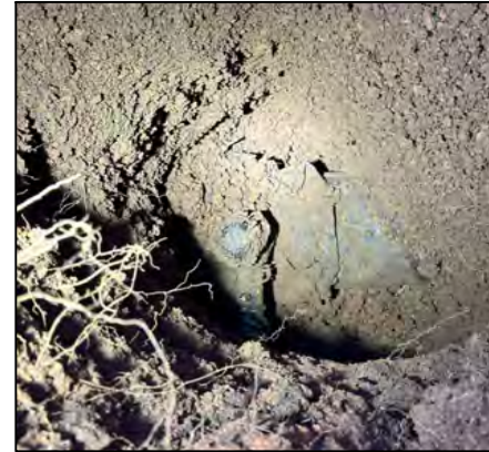
DOWN HOLE PHOTO OF UTILITY DATE: 08-03-2023
