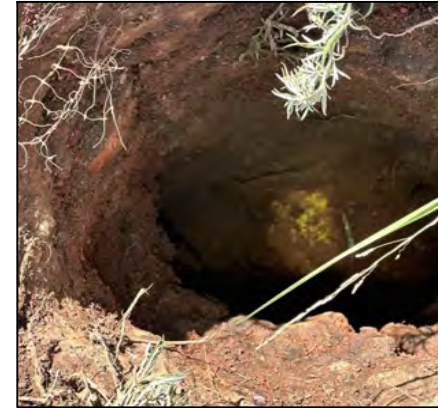
DOWN HOLE PHOTO OF UTILITY DATE: 08-08-2023
