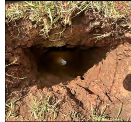
DOWN HOLE PHOTO OF UTILITY DATE: 08-09-2023
