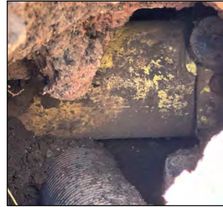
DOWN HOLE PHOTO OF UTILITY DATE: 08-03-2023
