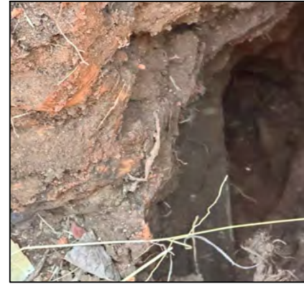
DOWN HOLE PHOTO OF UTILITY DATE: 08-08-2023
